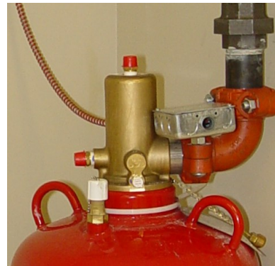
4. First thing—disconnect tank!
