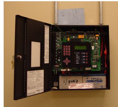
29. Have experience alarm technician, call out alarm system, silence building alarm, and cycle panel to activated any HVAC dampers connected to panel
